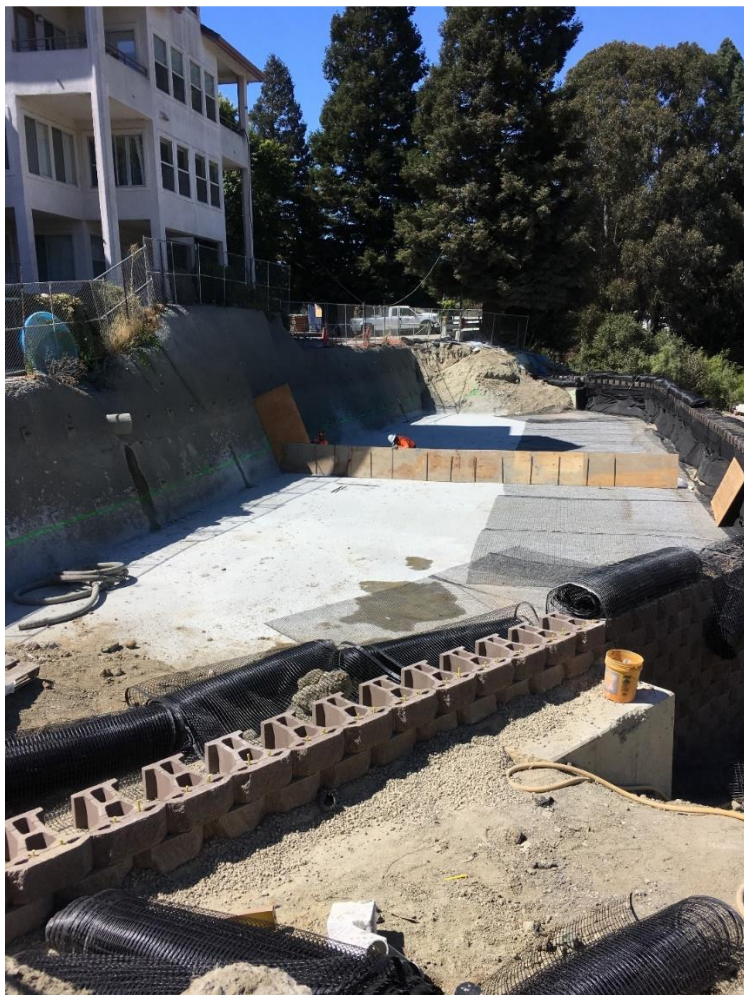
Figure 38 A section of the Bay Park Pinhole slide remediation project (Source: Cell-Crete Corporation).
