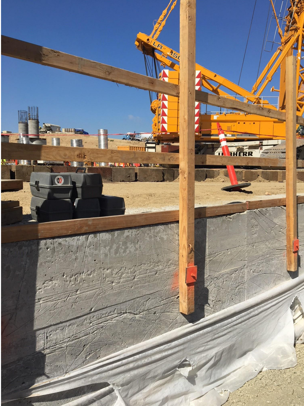
Figure 50 Closed view of the LCC at the Los Angeles Stadium (Source: Cell-Crete Corporation)
