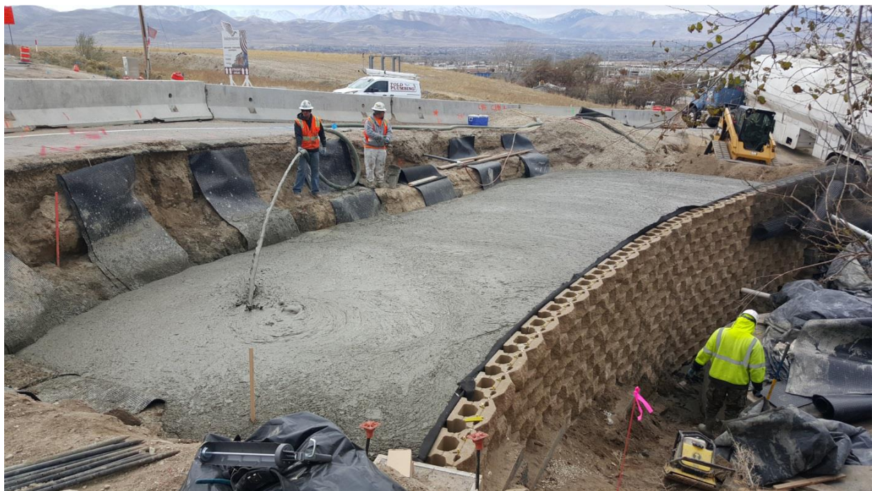
Figure 45 – Overview of the LCC MSE wall at I-15; SR-73 project. (Source: Gerhart Cole Inc.)
