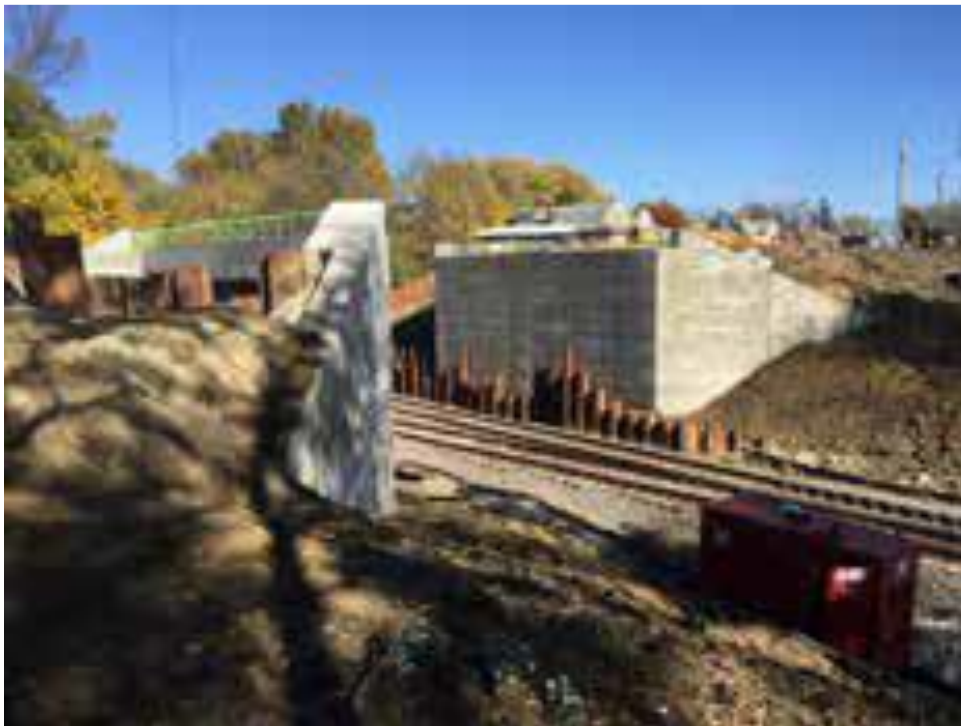
Figure 42 MSE wall built at Lynn Center Bridge Replacement project (Source: Aerix Industry)
