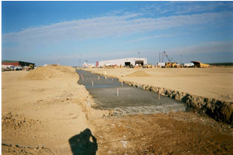
Figure 1. Picture of Fire Water Insulation near Fort McMurray.
