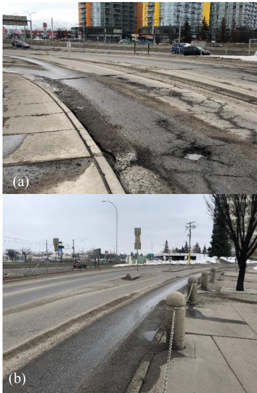
Fig. 1 Calgary bus lane in April 2018 (a) Traditional subbase lane and (b) LCC lane.
